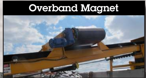
Overband Magnet The overband magnet ensures any metal is removed before material advances to the CBI secondary grinder.
